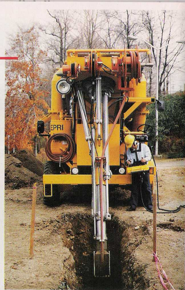
The Soft Trencher was designed for more efficient and environmentally safe excavation.
