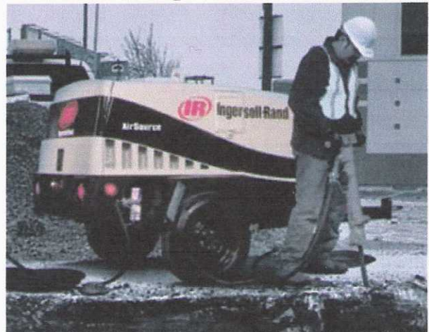
Ingersoll Rand AirSource Compressors
